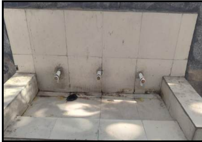
Poor cleanliness and hygiene issues.
