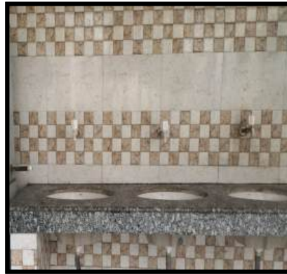
Water Station with multiple taps
